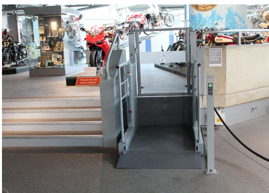
Fig. 11 – Lift for steps on mezzanine level
